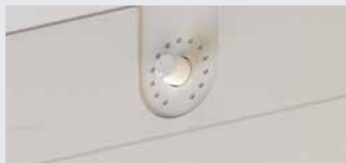
Rotary dimmer control
